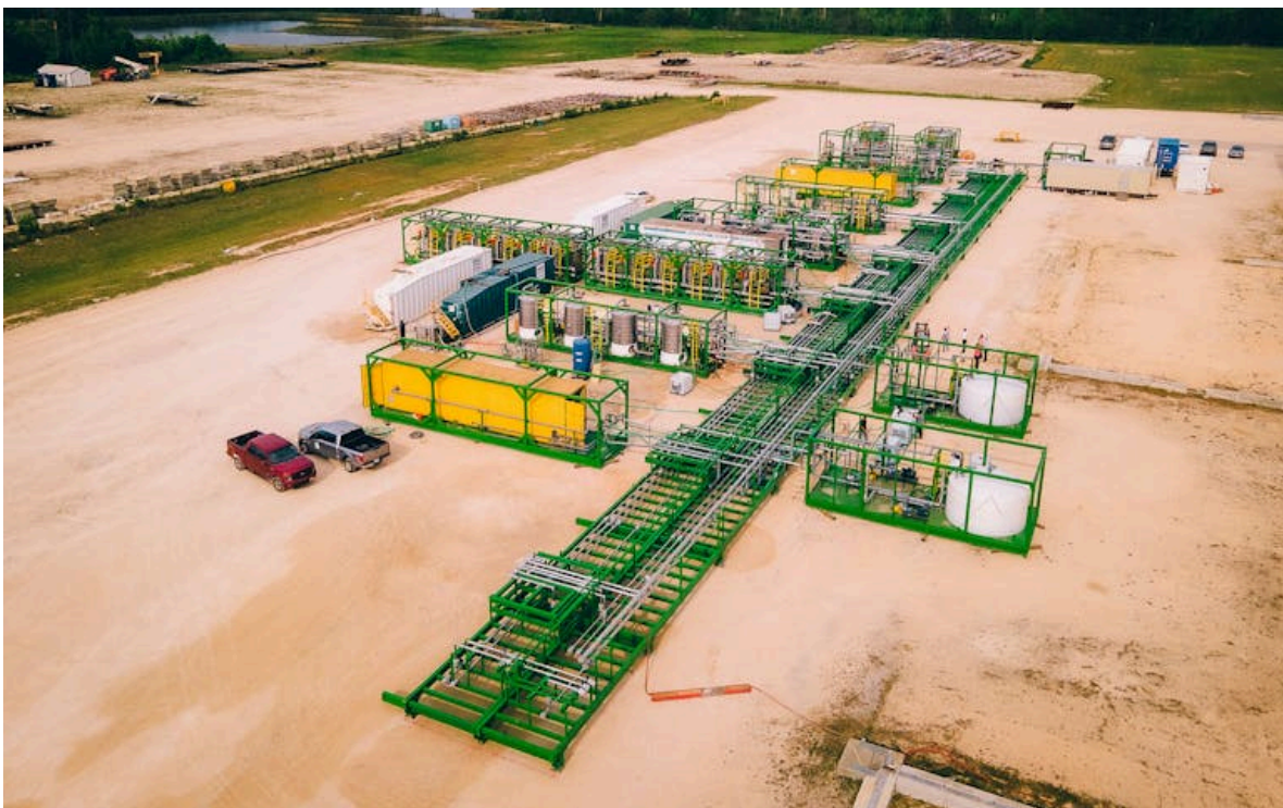
An aerial view of International Battery’s modular DLE system in Lake Charles, Louisiana. Courtesy of International Battery Metals
